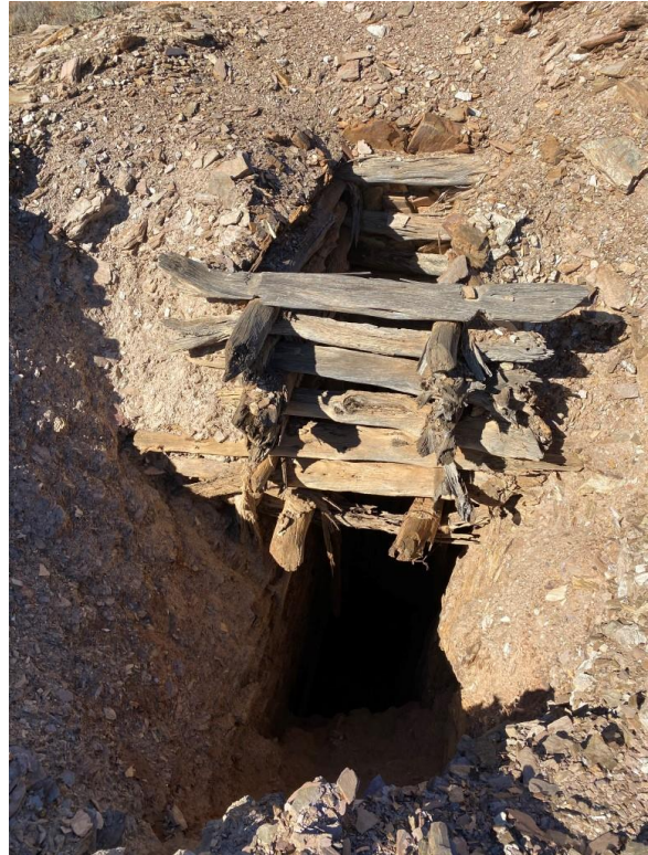
Typical shaft, partially collapsed due to argillic alteration
