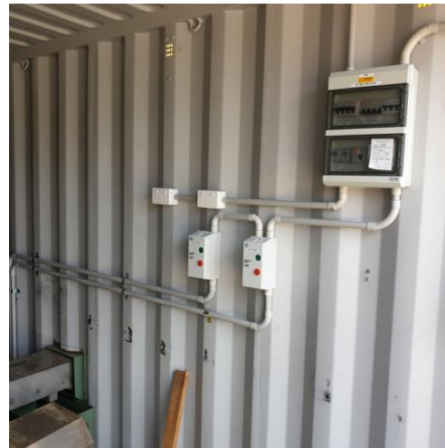
Sortex unit has all new wiring and trip switches
